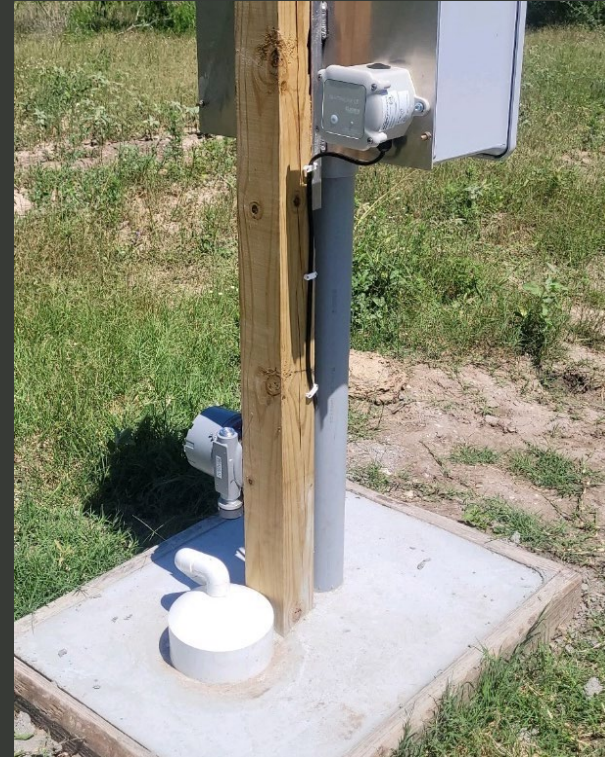
Sensor location (on post by vent tube)
