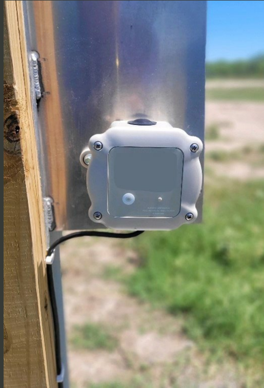
2-channel cellular monitoring system
