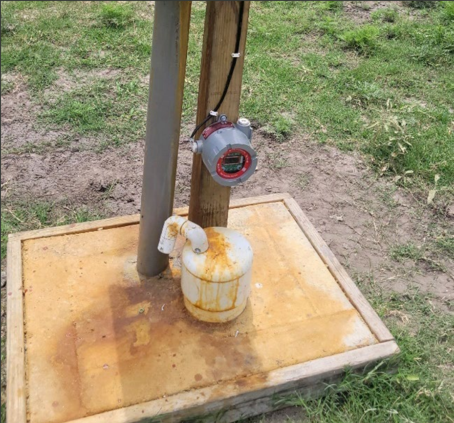
Discoloration, residue, and corrosion from chlorine emissions
